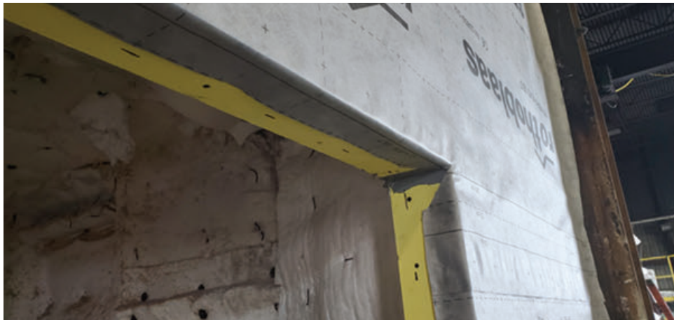
FIGURE 5: Test 1 setup – Close-up of gypsum board to window edge and WRB wraparound
