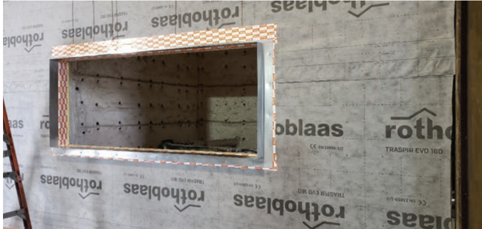
FIGURE 6: Test 1 setup – Installation of window frame surround and sealing tape prior to mineral wool overlay
