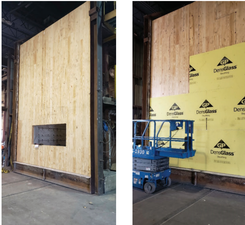
FIGURE 3: Test 1 setup – CLT wall completed in frame (left); installation of fire-rated gypsum board (right)
