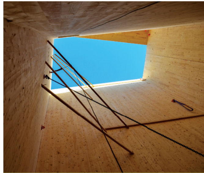
CLT shaft walls were chosen for the University of Massachusetts (UMass) Design Building in Amherst, MA in part to demonstrate that mass timber building elements can replace traditional building materials for a number of applications, including shafts.
