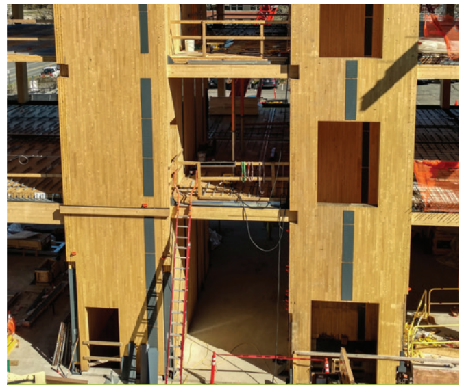
For the four-story UMass Design Building, the CLT shaft walls doubled as shear walls, providing lateral load (seismic and wind) resistance.
