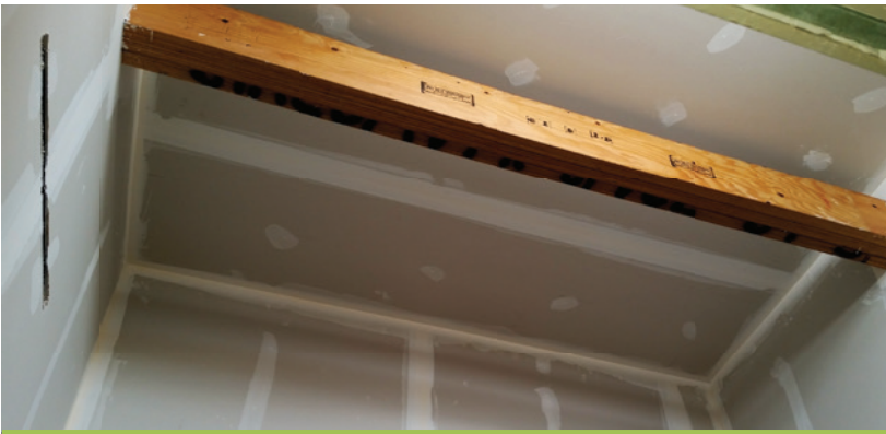
Wood-frame elevator hoist beam
