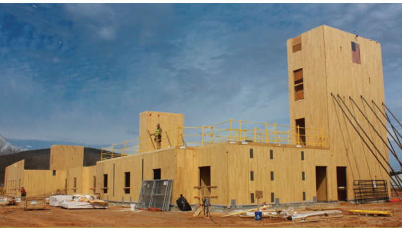
One of the benefits realized from the use of CLT shaft walls at Redstone Arsenal was speed of erection. Each of the shaft walls was a single, 37.5-foot-long piece.
