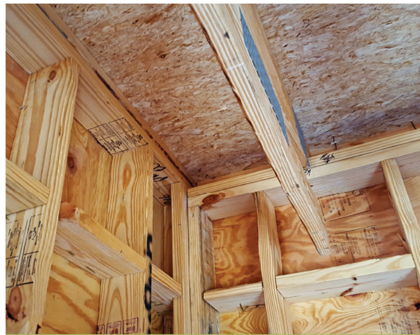
Example fire barrier wall continuity, extending to underside of floor/roof sheathing above
