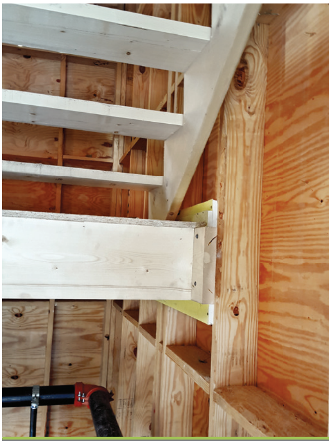
Stair landing framing attached to shaft wall through two layers of gypsum prior to landing beam hanger installation
