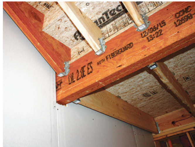
Stair landing beam shaft wall structural penetration prior to firestop system installation
