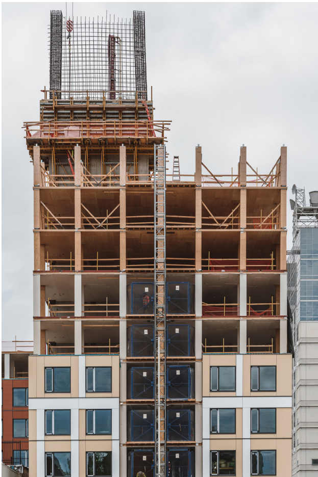
1510 Webster – Oakland, CA oWOW / One story of steel over 16 stories of mass timber over a two-level concrete podium
