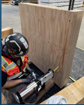
THE EPOXY IS A TWO-PART SYSTEM THAT UTILIZES THE SAME CI-GV EPOXY. THE FIRST PART IS APPLYING A THIN GEL COAT AROUND THE ENTIRE PERIMETER OF THE HOLE THAT REQUIRES 24 HOURS OF CURE TIME.
