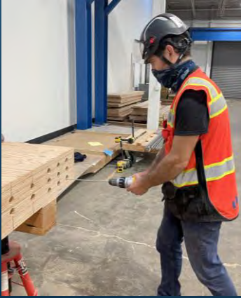
1 ¼" TENSION ROD HOLES WERE MACHINE FABRICATED TO CREATE A PILOT HOLE AND THEN HAND FABRICATED TO THEIR FULL 33" DEPTH.
