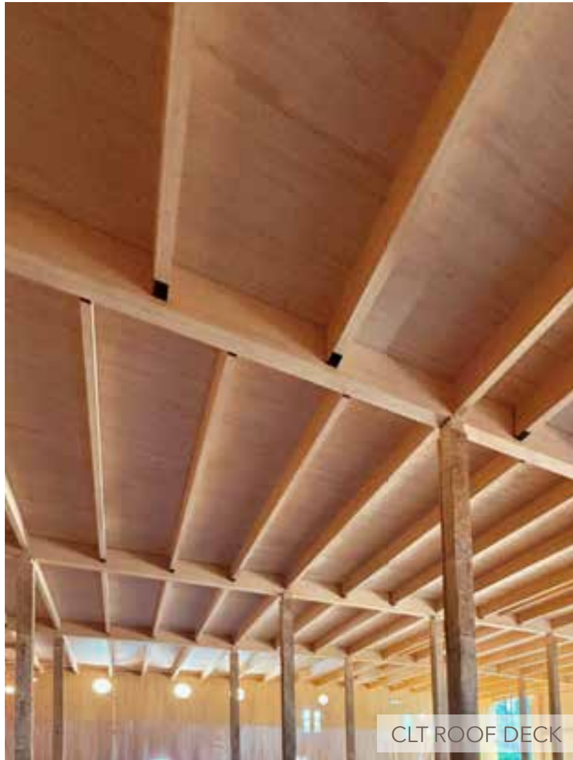
GLULAM BEAMS + COLUMNS
