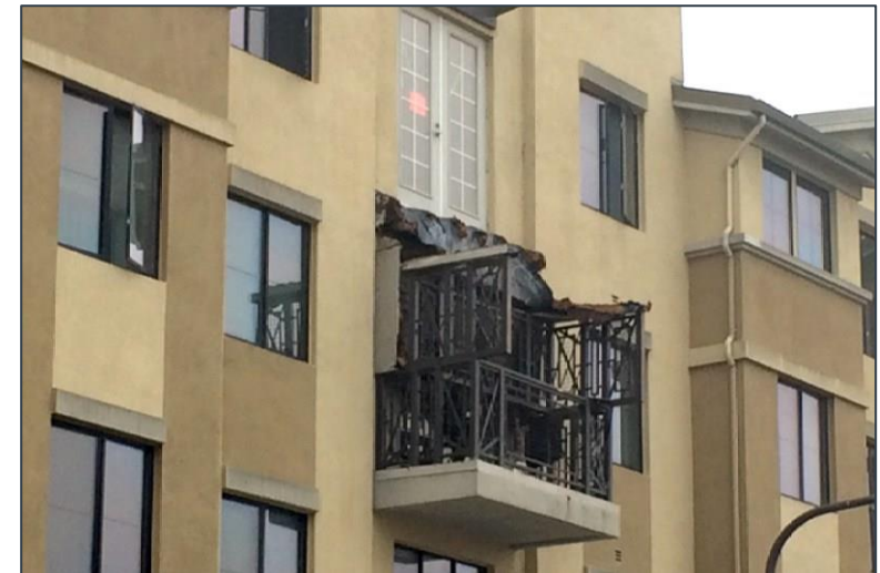
Aftermath photographs of the collapsed balcony – Emily Dugdale & San Francisco Chronicle
