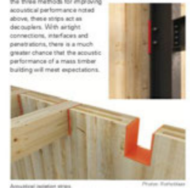
Acoustical isolation strips
