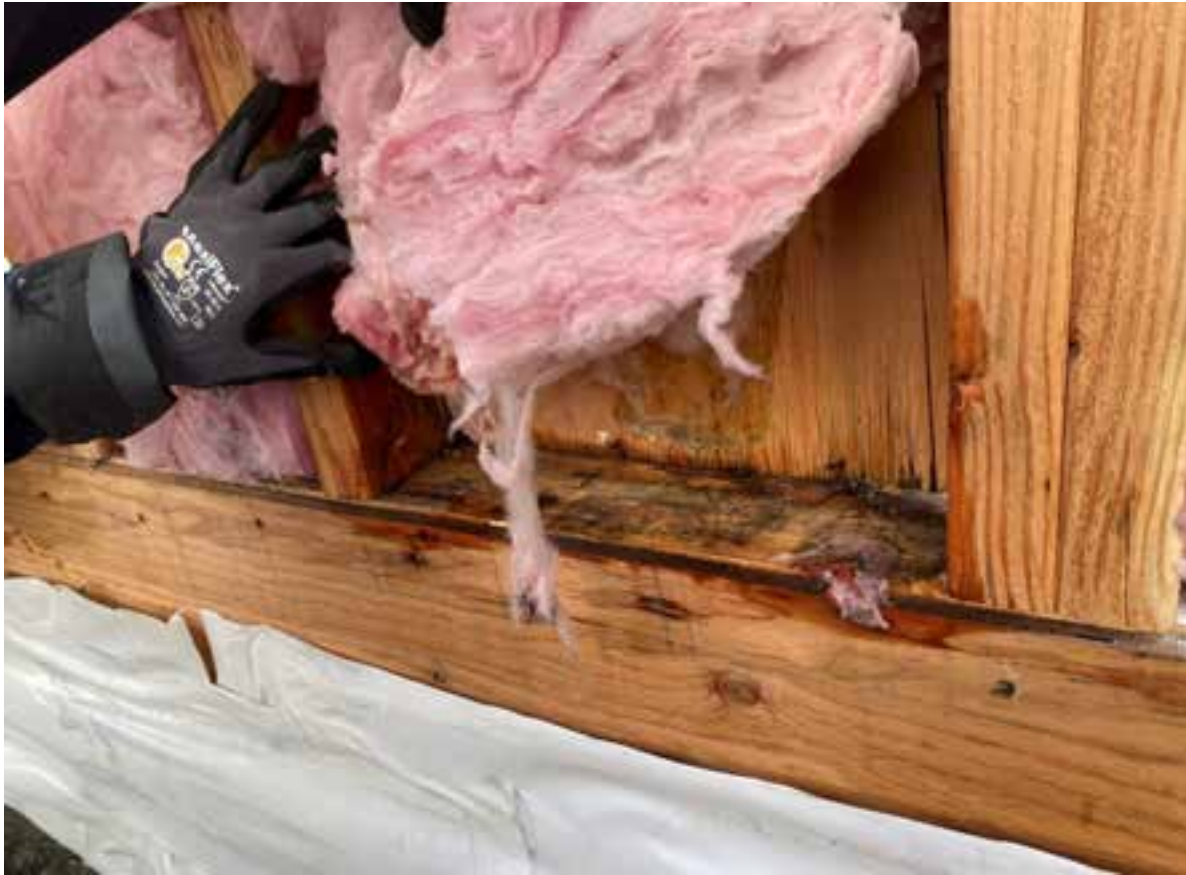
Moisture accumulation at stud bays, organic growth present, limited drying potential due to shrink wrap
