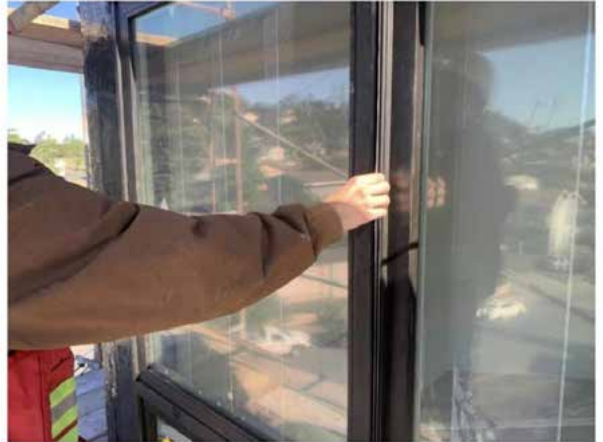
Photo 12.1f - Operable window with minimal compression of gasket. Unit 412 west elevation
