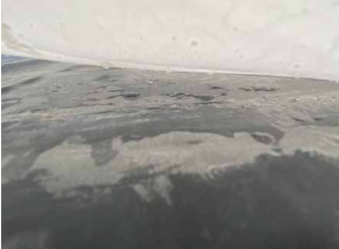
Leak through shrink wrap onto EPDM temp roof membrane
