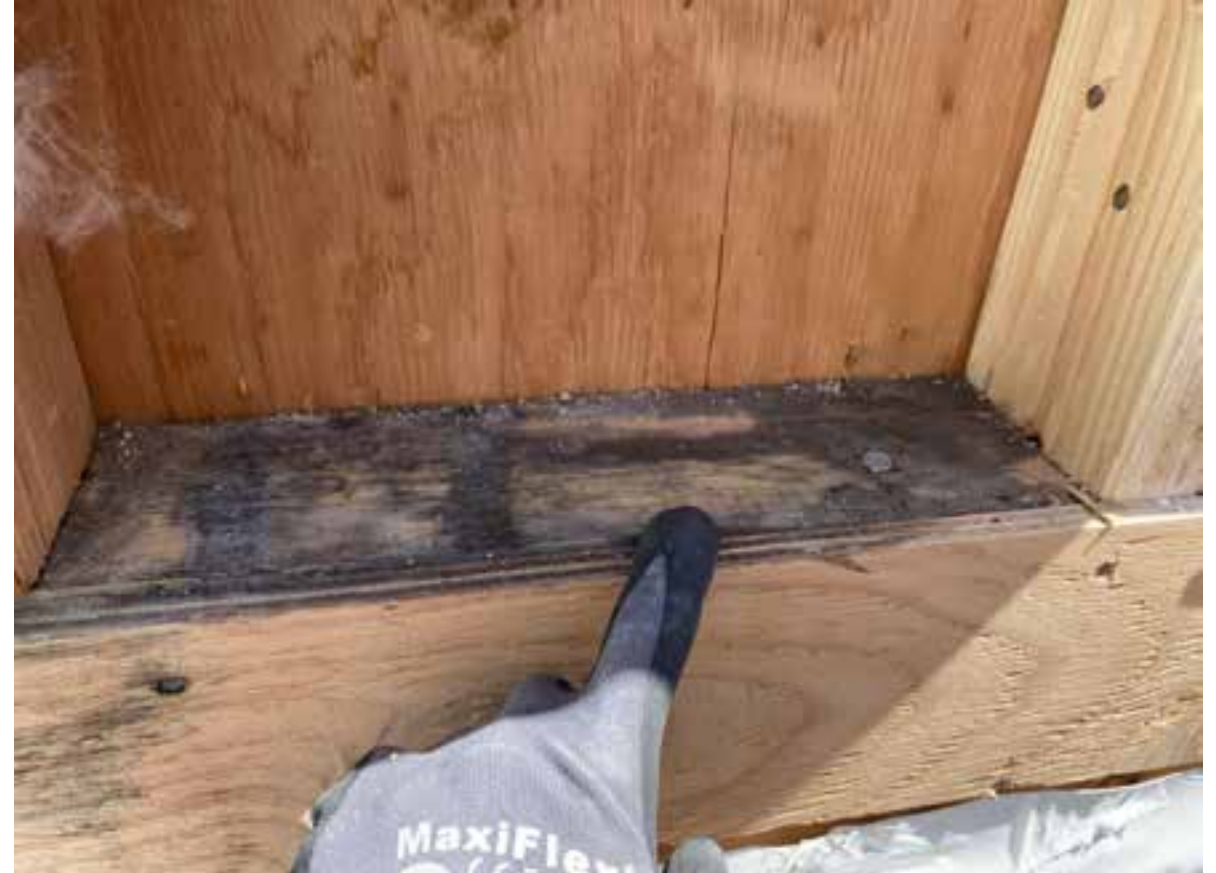
Moisture accumulation at stud bays, organic growth present, limited drying potential due to shrink wrap
