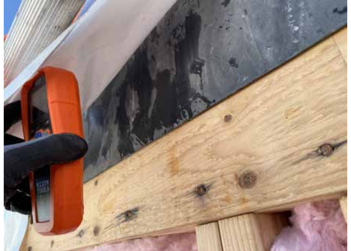
Water draining off EPDM temp roof membrane down unprotected side walls of mods, behind shrink wrap
