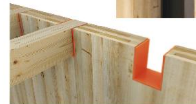
Acoustical isolation strips
