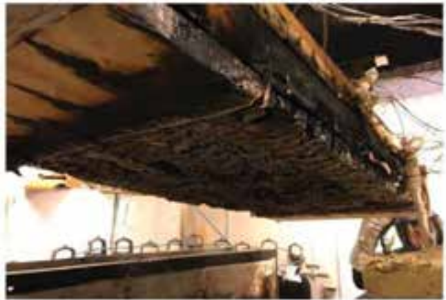
Fire Safety Challenges of Tall Wood Buildings – Phase 2: Task 5 – Experimental Study of Delamination of Cross Laminated (CLT) Timber in Fire
