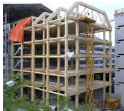
Tamedia post and beam structure Architecture by: Shigeru Ban Photo credit: Blumer-Lehmann AG
