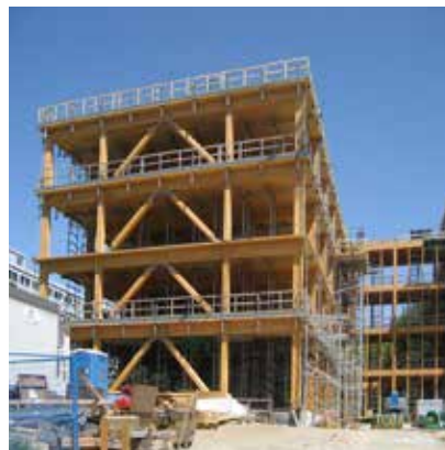
Exposed view of glulam chevron braces at UBC Earth Sciences Building Architecture by: Perkins+Will Photo credit: Equilibrium
