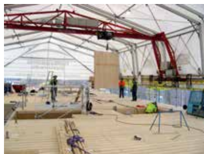
Weather protection at Limnologen. Moveable rising tent structure. Photo credit: Johan Vessby
