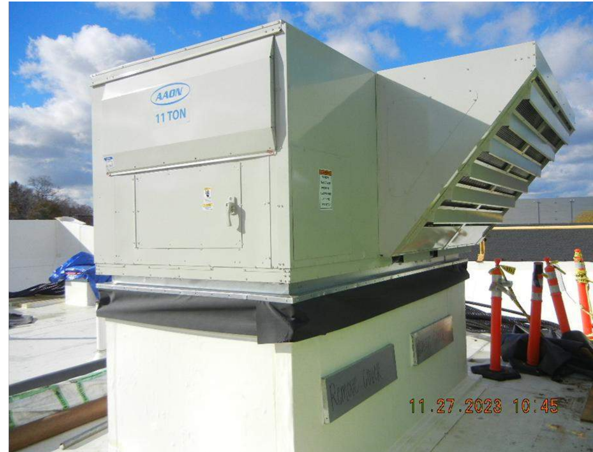
ERV – Energy Recovery Ventilator
