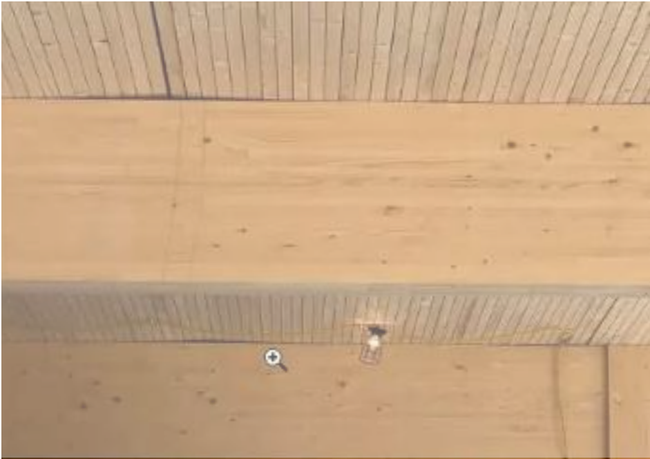
Moisture issues if not enough gap
