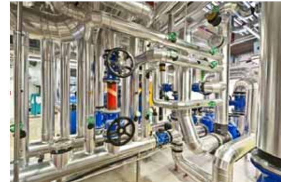
Mechanical room in the basement
