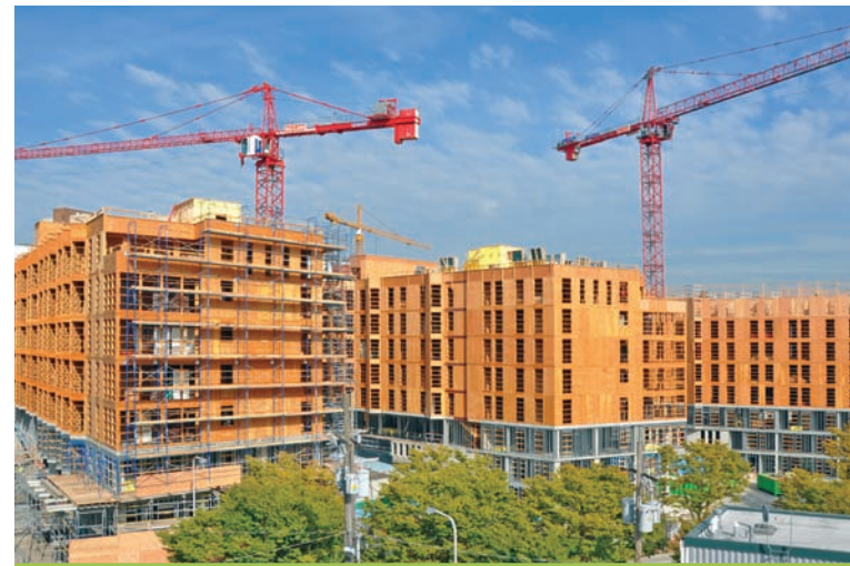
Multi-level podiums were added to the 2015 IBC, but require an AMMR under previous versions. This University of Washington student housing development was built under the Seattle Building Code, which permitted multi-level podiums years before their adoption in the 2015 IBC.
