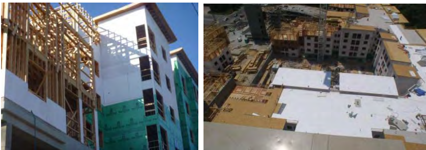
2-hour rated wall assembly with FRCC OSB in Type III construction (Student housing, College Park, MD)
